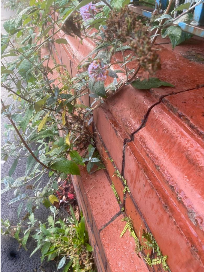
Buddleia growing between masonry
